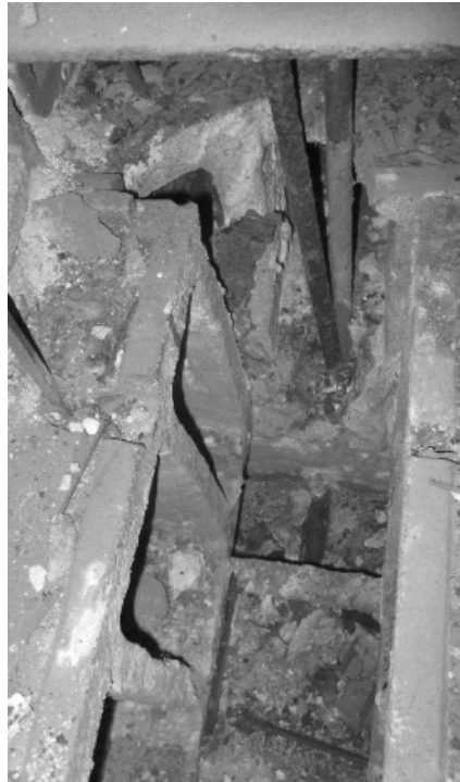
Condition of original 'J hooks' supporting the original scroll brackets
