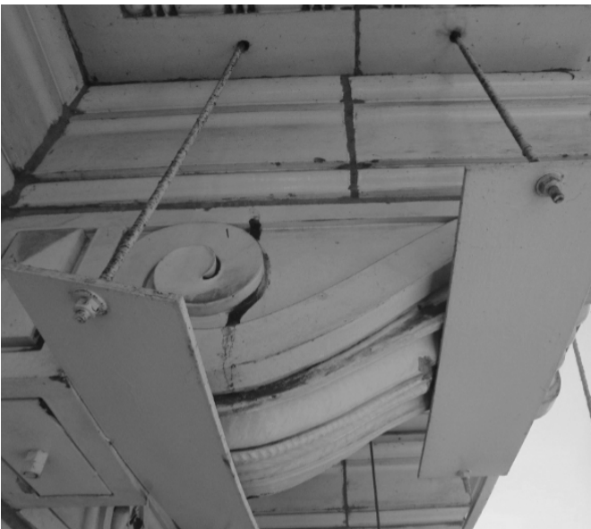
Temporary support on cracked original terra cotta scroll brackets
