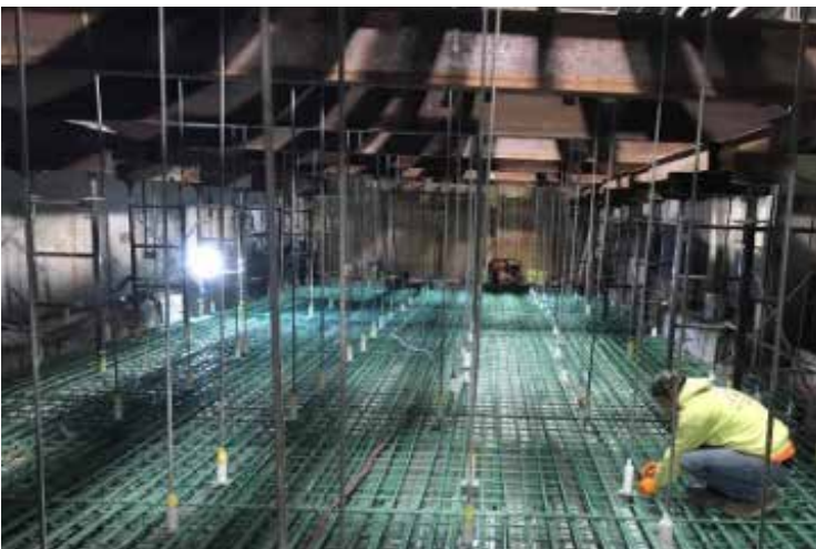
Figure 3. Installation of new reinforcing steel for structural slab repair at an interior driveway with hanger rods supporting the plenum slab below. This location is over active rail lines.
