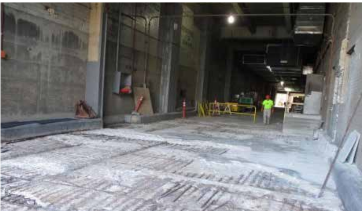
Figure 2. Structural slab deterioration at interior first floor driveway over active rail
