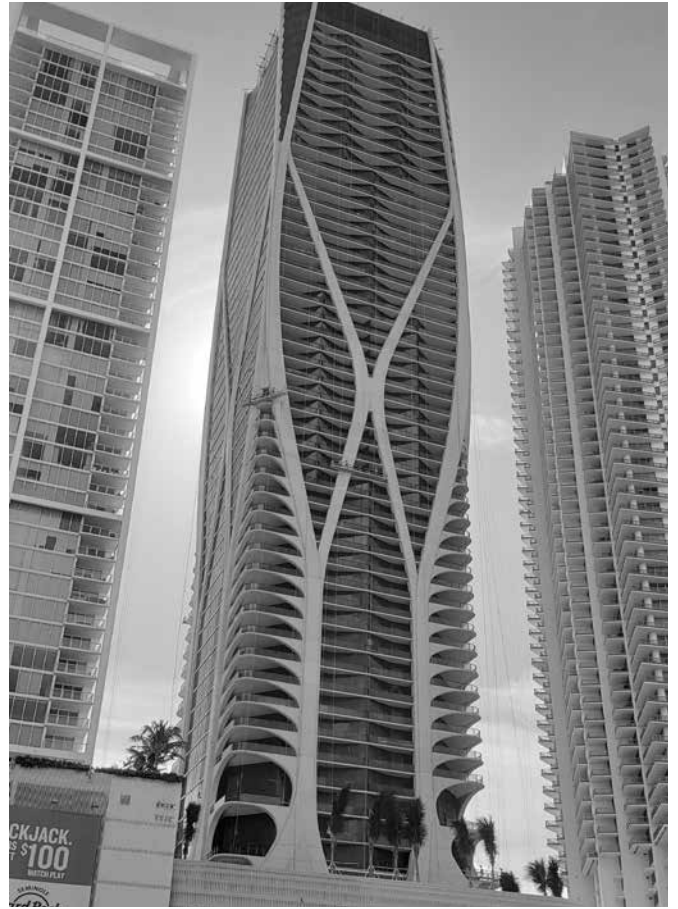
Figure 5: Sky Stage Ultra (SSU) suspended access platforms navigate around exoskeleton sections of One Thousand Museum.
