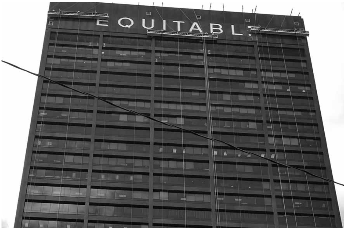
Figure 4: The suspended access project at 100 Peachtree earned Sky Climber the 2019 SAIA Project of the Year Award
