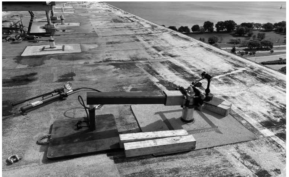
Figure 6: View of a typical lateral pull load application with chain hoist test arrangement.
